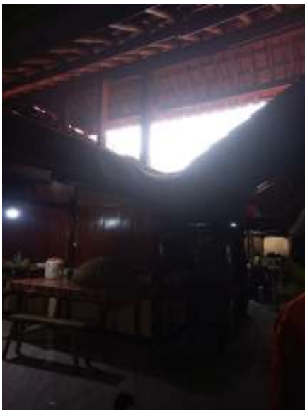
Picture 8 air holes House of Mr Supriyadi
